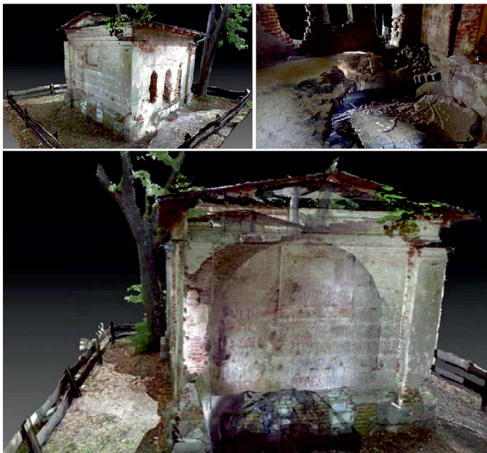
Fig. 2. 3D model of the Rutkowski family’s burial chapel in Pasym, developed on the basis of a point cloud from ground-based laser scanning (author of the project: Paweł Kondraciuk, 2018 – Regional Digitization Workshop, Elbląg)
