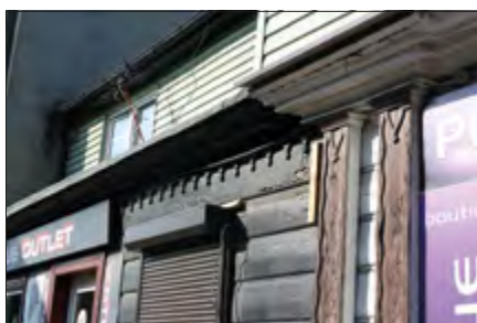
Fig. 5. Decorative boarding on the façade of the building at 15 Długa Street (source: the collection of the D.O.M. foundation).
