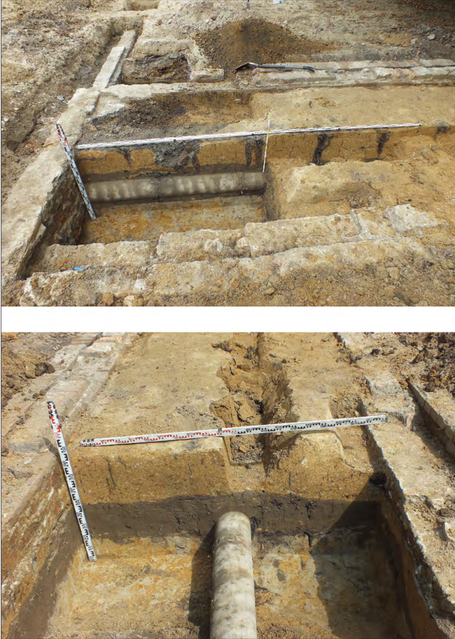
Fig. 10. The inside of block no. 6 (item 9), A–B and E–F profiles, a view of a concrete drain pipe (photograph by W. Tabaszewski).
