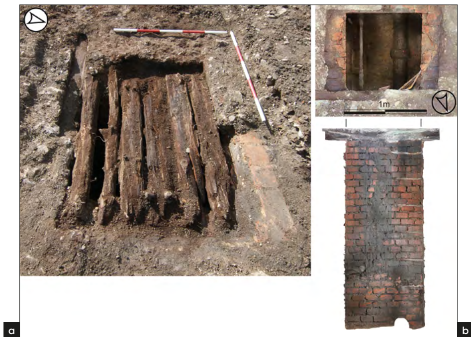
Fig. 10. Revision shaft at the camp sewerage close to the kitchen building: (a) temporary covering of the shaft with secondary used beams that were poured with a thin cement mixture, which is already removed on the field photograph (photograph by D. Pilař); (b) plan and southern profile of the shaft.
